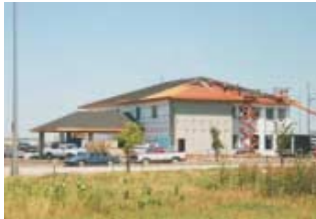
At right: Standing seam roof work just getting started at the Choice Financial job site in Fargo, N.D.
