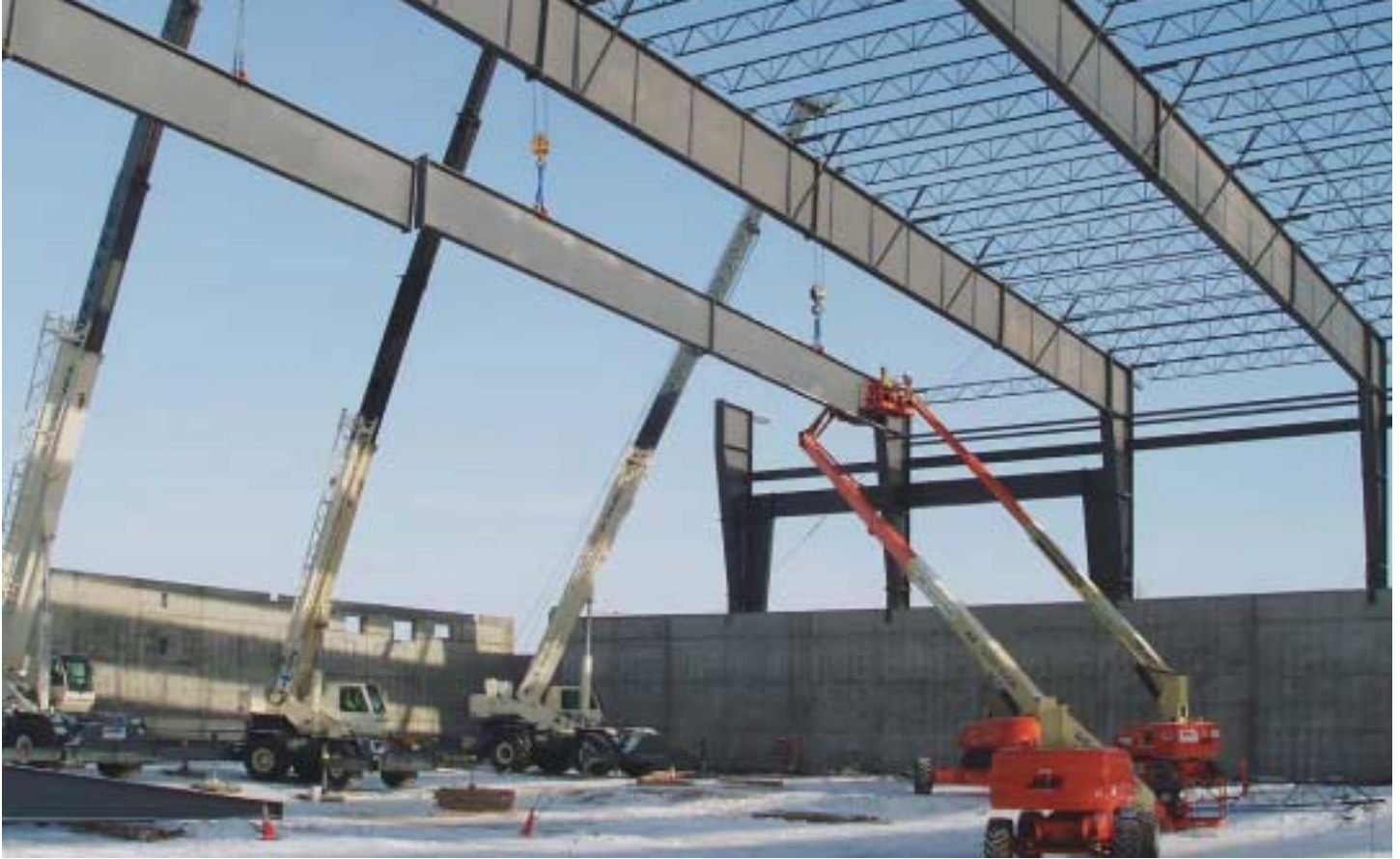
Three cranes are required to hold and stabilize each frame during erection.
